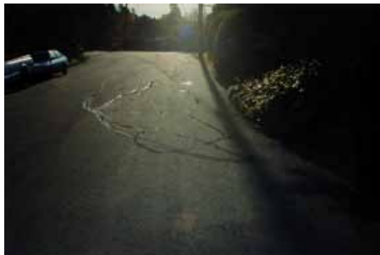
Figure 6 (above): View to the southeast along Highgate Road. The residence at 18 Highgate Road is to the right. Note arcuate cracks in the asphalt, which represent small-scale deformation within the Blakemont landslide.
