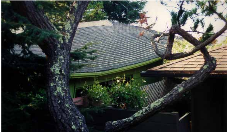
Figure 5: View of landslide-induced distress to the residence at 18 Highgate Road. Note the warped roof and cracks along the side of the residence.
