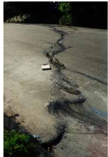
Figure 7 (right): View to the south across Highgate Road near 16 Highgate Road. Crack in asphalt is up to 3 inches wide. A driver of a car passing by while I took this photo said that the road was resurfaced two years ago. Clipboard for scale.
